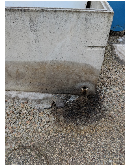
8) Diesel staining near stormwater drain from diesel ASTs
