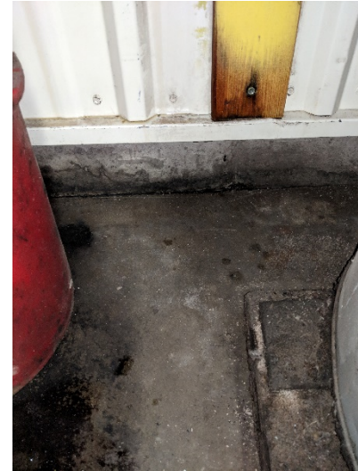
10) Oil staining near floor and wall joint – maintenance shop
