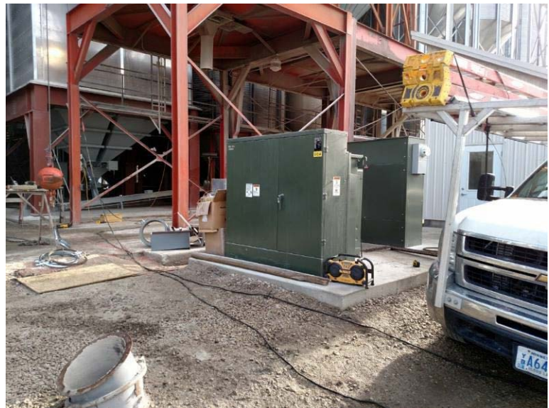
PHOTO 27. East Elevator transformer viewing southeast.
