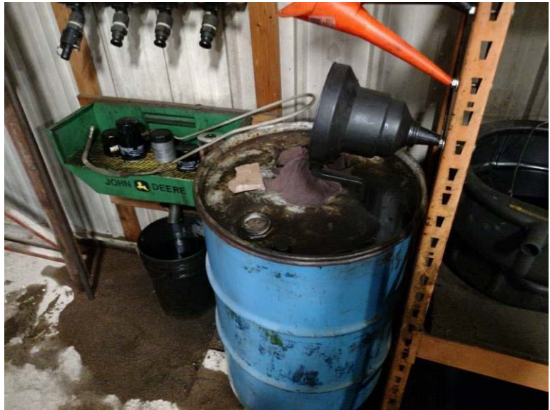
PHOTO 42. Used oil collection in maintenance building.
